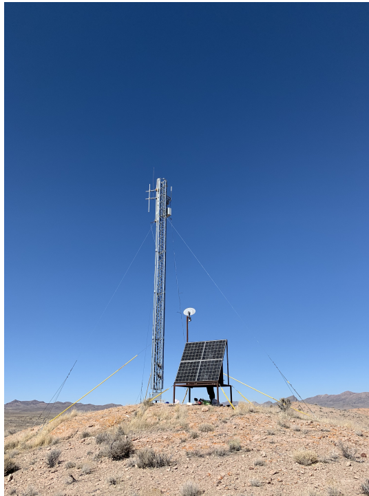
FIGURE 2.22: Photo of the Middle Drum Communication Tower. The batteries and electronics that controls the TALE SD DAQ are installed at the back side of the solar panels. The wireless antenna to communicate with the SDs is install at the top of steel tower.
